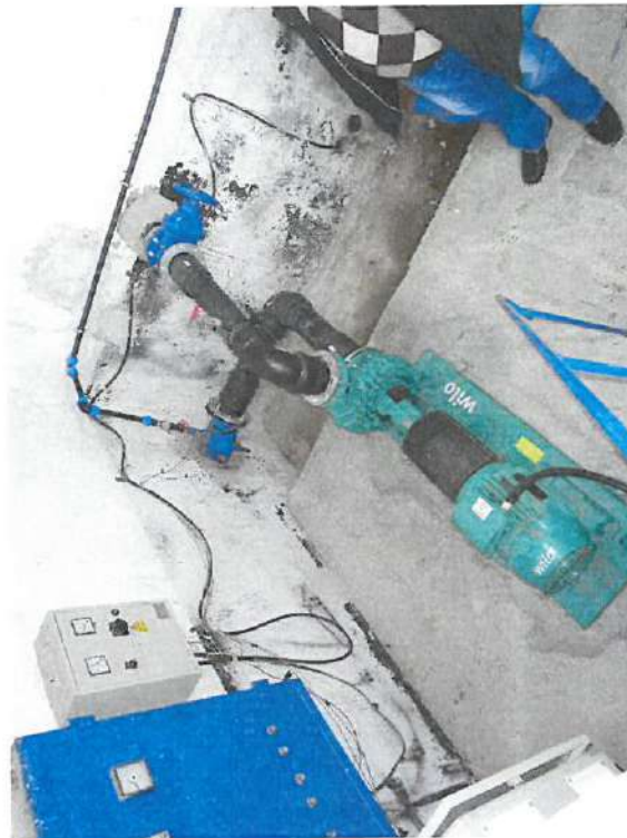
Foto 16: Interior casa pompe cheson capture.
